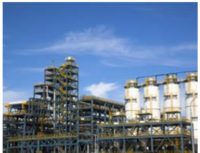
Equipment support structure
